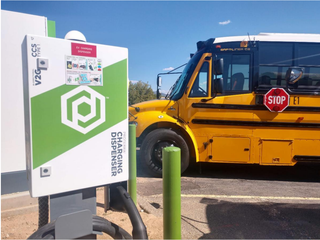
Santa Fe Public Schools EV bus charging station. Photo courtesy of PPC Solar.
