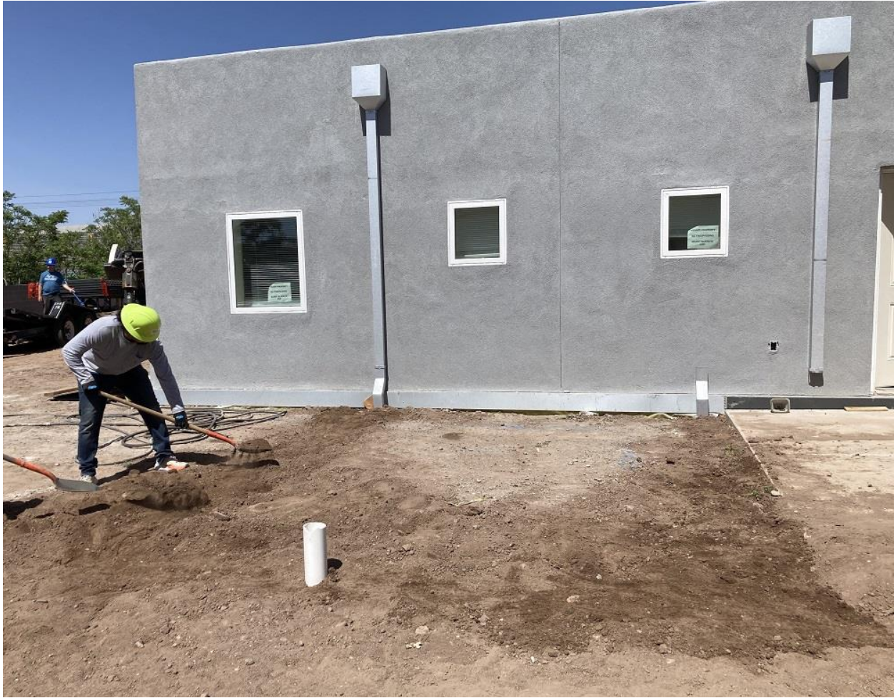
CUTLINE: Several New Mexico Mortgage Finance Authority (MFA) employees volunteered on May 22, 2024, to help build new homes being constructed by Greater Albuquerque Habitat for Humanity. MFA Green Initiatives Manager Dimitri Florez assisted with fitting and installing PVC pipe and backfilling the trenches. (Photo courtesy New Mexico Mortgage Finance Authority)
